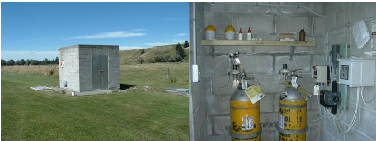
Figure 11-2: Fairlie WS Treatment Plant
