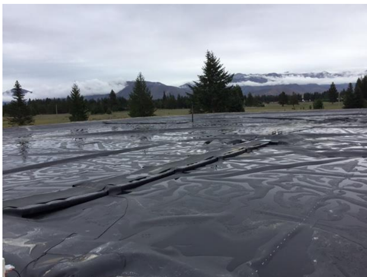
Figure 11-19: Twizel WS Raw Water Reservoir
