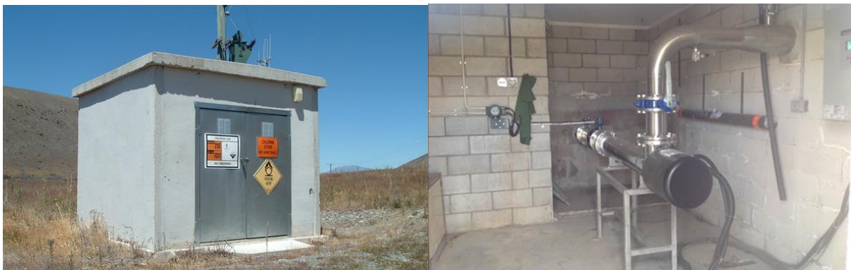
Figure 11-10: Lake Tekapo WS \text{Cl}_2 building & UV treatment
