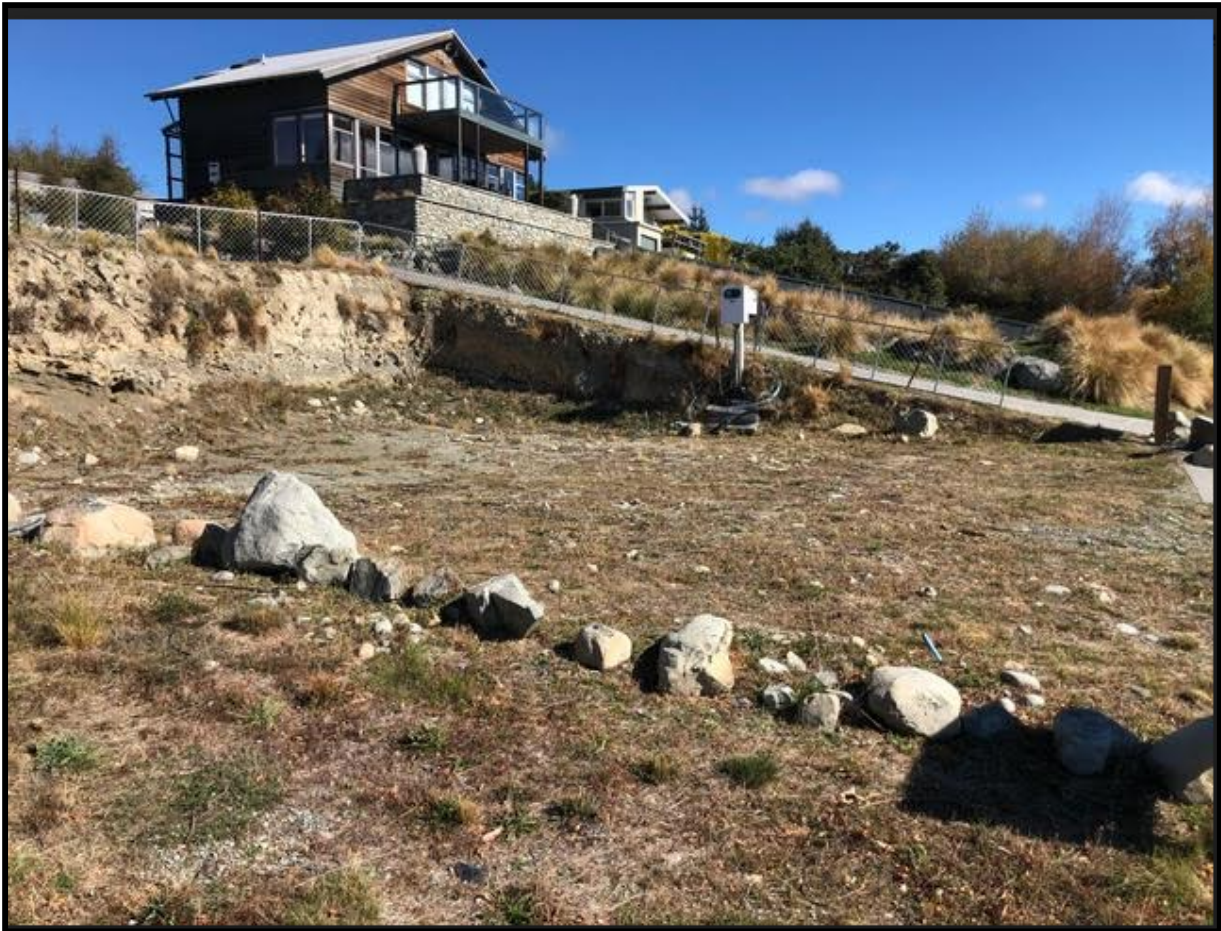
Figure 7 – The subject site after 2018 earthworks in its current state. Opposing submitter’s dwelling is shown in the far ground
